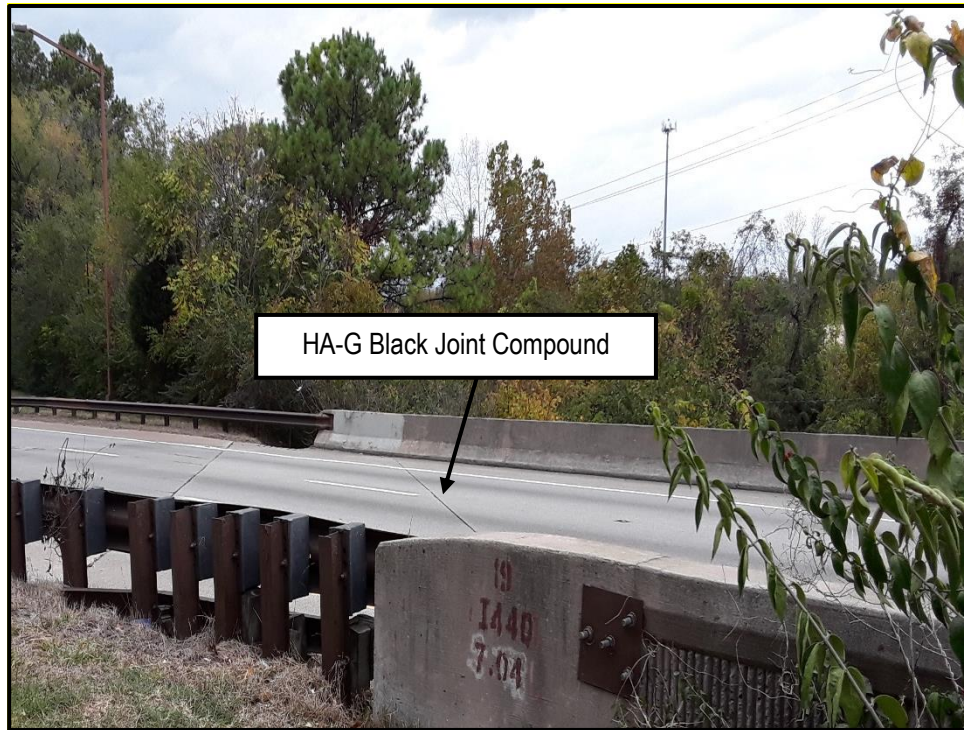
Photo 7: View of HA-G on the westbound I-440 bridge over Glenrose Avenue and CSX RR
