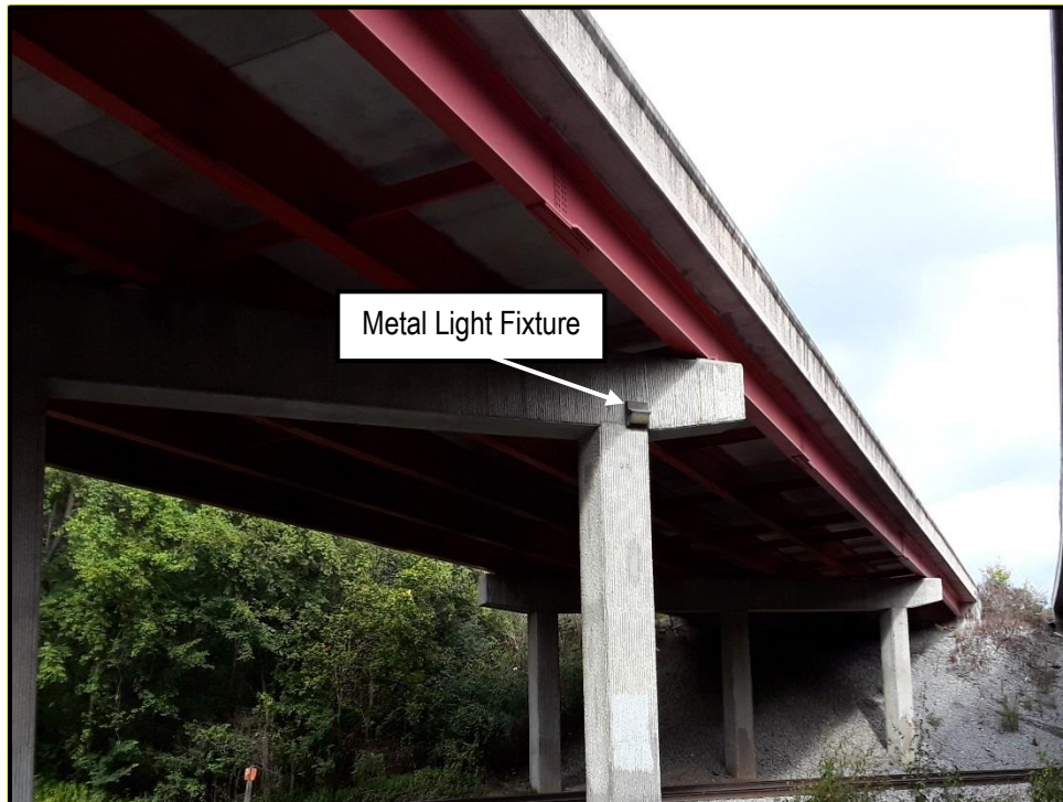
Photo 8: View of metal light fixture on the westbound I-440 bridge over Glenrose Avenue and CSX RR
