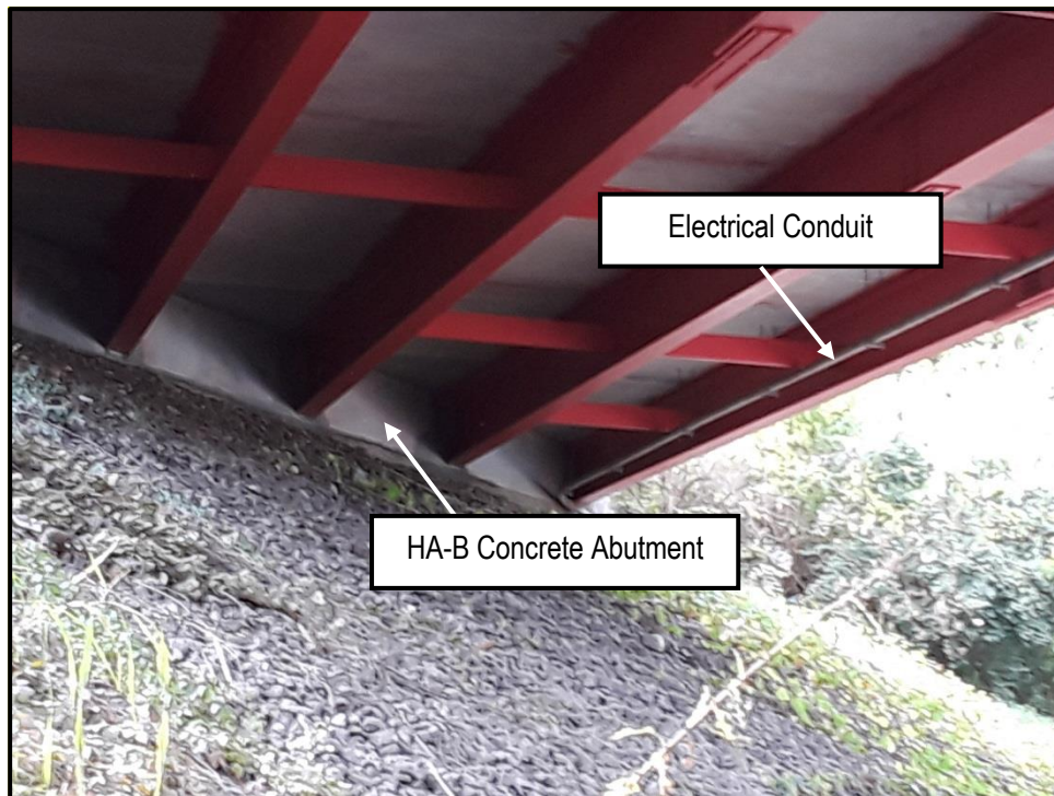
Photo 2: View of HA-B on the westbound I-440 bridge over Glenrose Avenue and CSX RR
